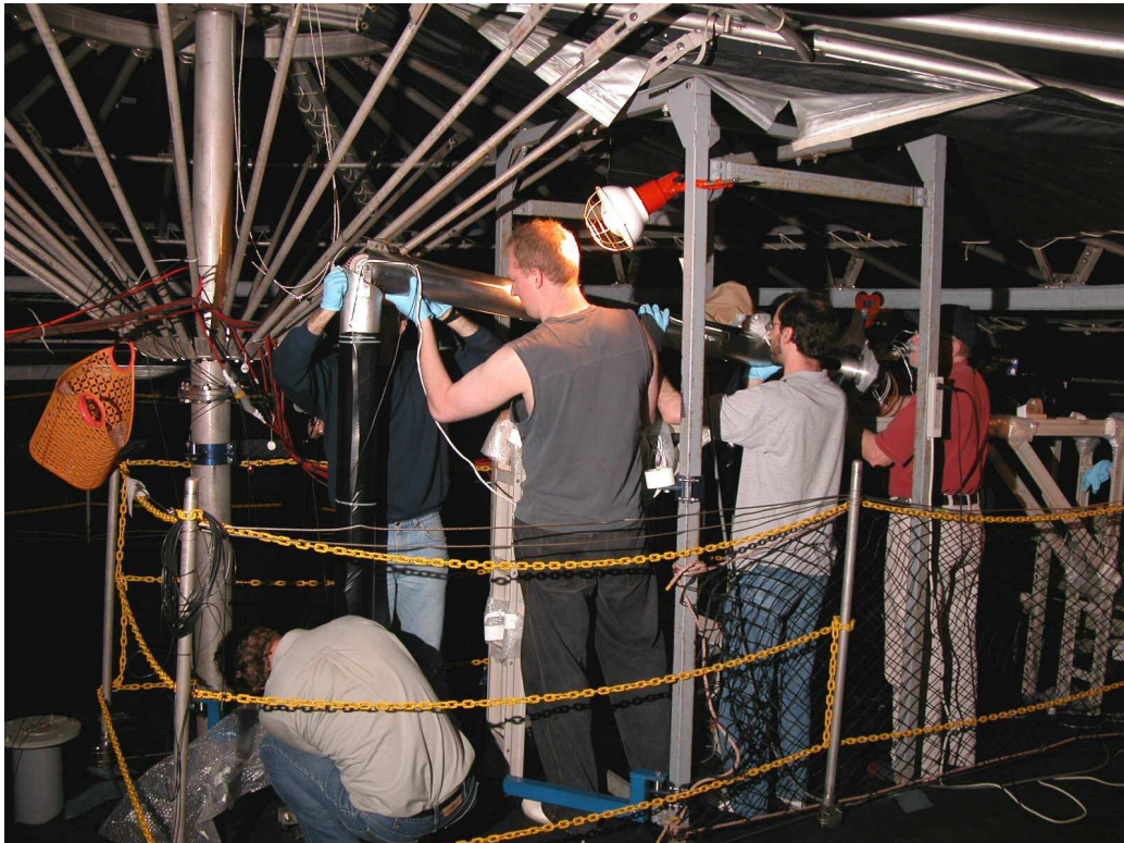
Figure 3.18: Before lowering part 2 of the VS into the 1KT the clamp holding parts one and two straight must be fastened.
